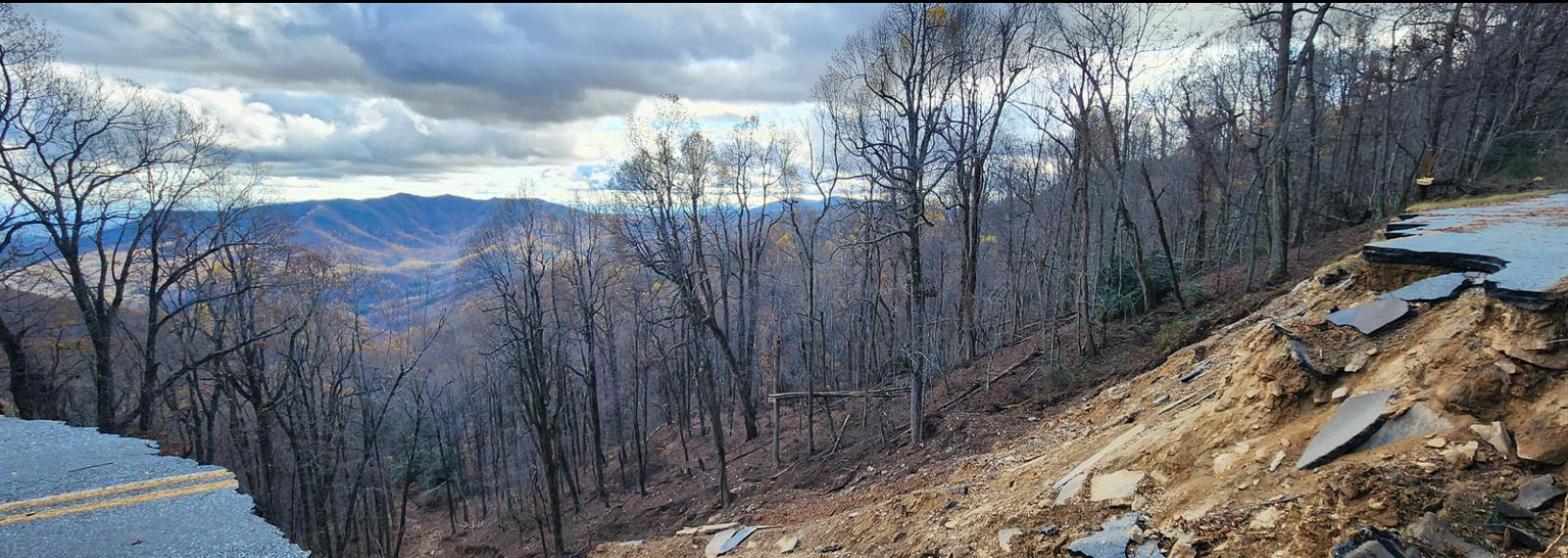
Photo caption: Collapse of roadbed and slope at milepost 337 near Gooch Gap, NC. NPS Photo.
